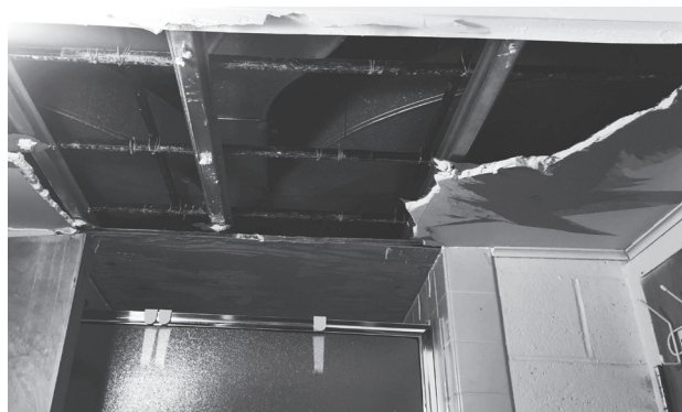
The bathroom ceiling to room 218 in Hart fell in after a water leak on Friday, Nov. 8.
